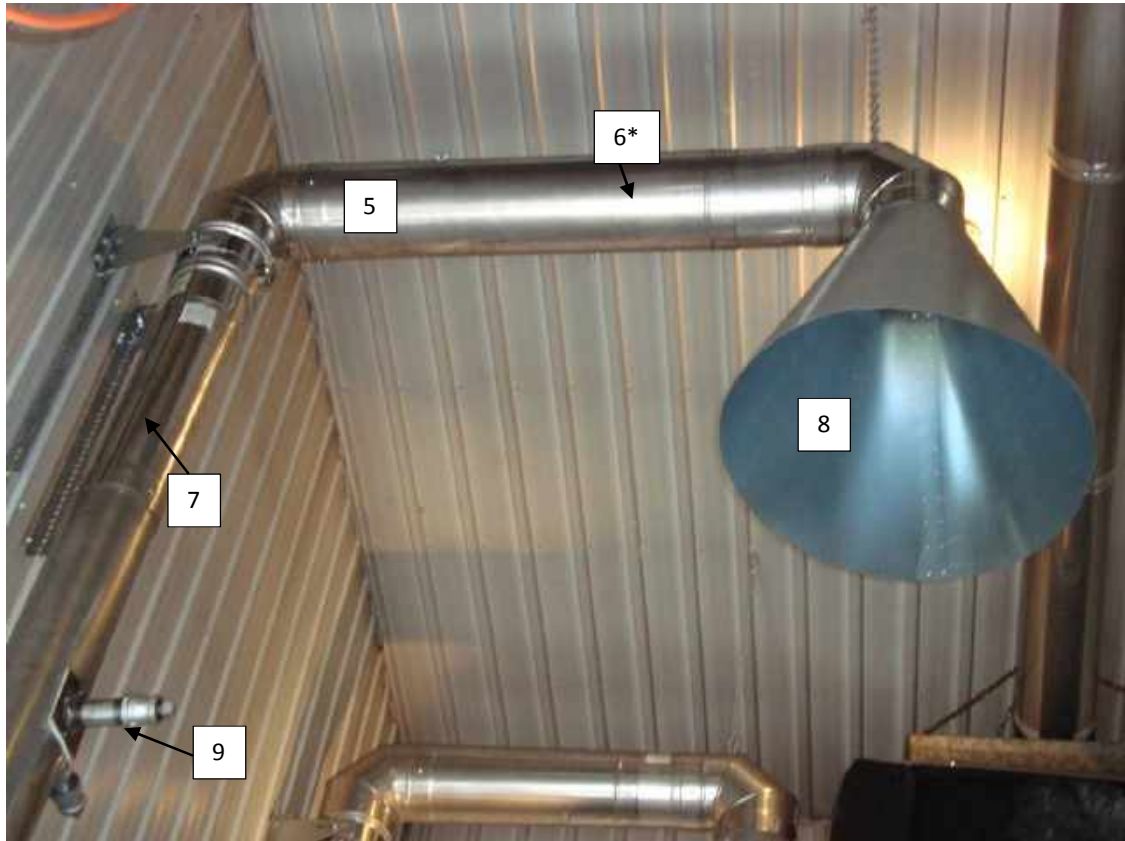
Picture 2 : Hood and mixing baffle
